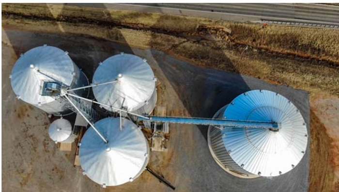
Sweet® enclosed belt conveyor installed at Gunter Peanut Co. in Binger, OK.
